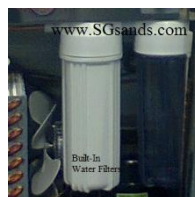
Built-In Water Filters Inside Cooler
